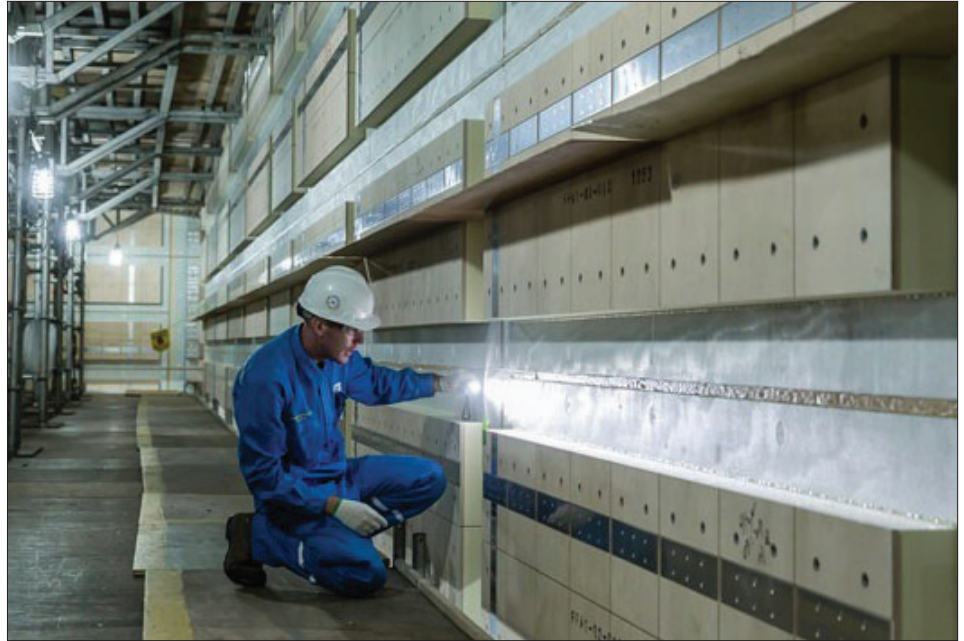
Panel inspection of GTT's Mark III membrane containment system. Image: GTT/Roland Mouron
