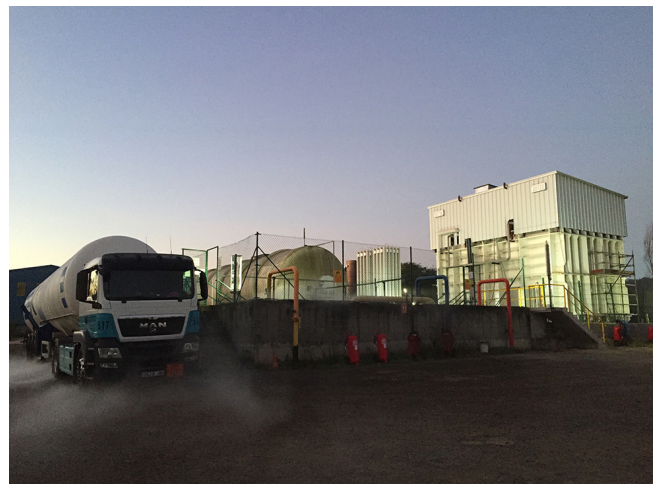
Figure 1 : LNG facility located in UNEMSA factory, Spain
